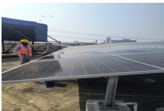
Cleaning of Solar Panels (NSSTA)
