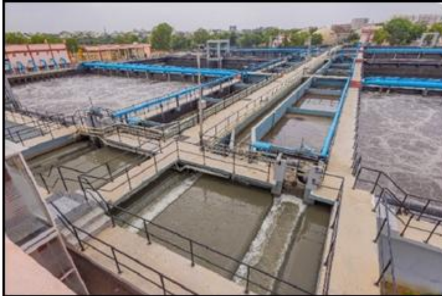
Water Treatment at Dehlawas Plant
