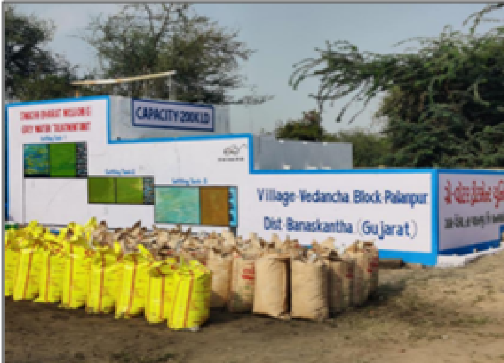
Image 3: Greywater Treatment Plant in Vedancha
