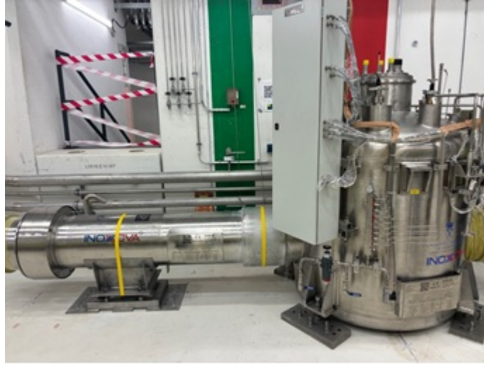
Fig 3: Cryogenic component from INOXCVA at FAIR site
