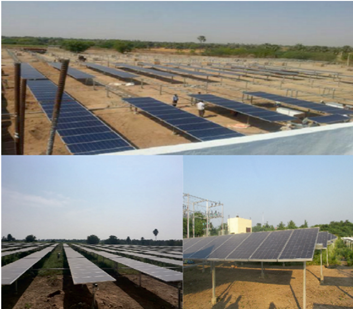
Solar Power Plant
