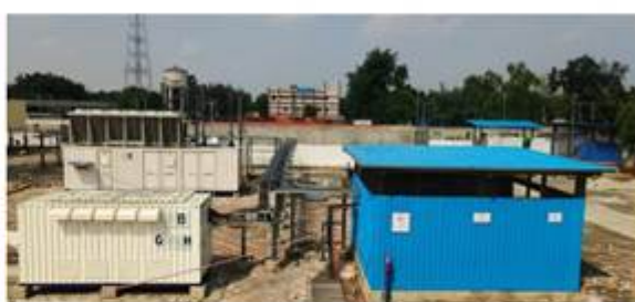
View of Hydrogen Facility
