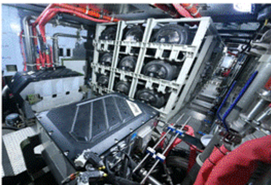
Fuel Cells & Hydrogen Cylinders
