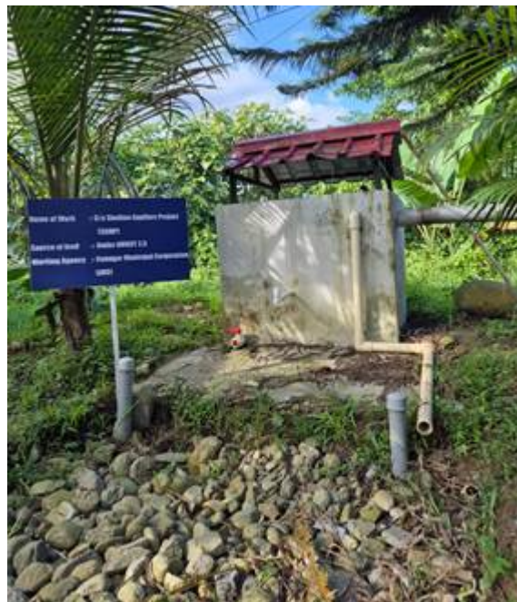
Recharge pit with storage tank facility for rooftop rainwater harvesting in Itanagar
