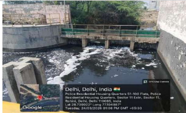
Functional but inadequate due to overflow observed in June, September, October, November 2025 and January 2026
