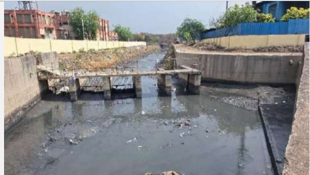
Functional but overflow observed. Also, huge sludge deposited upstream of tapping arrangement and screens broken
