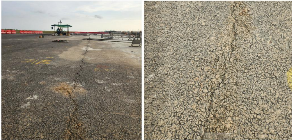
Figure 9: Cracks at Parallel Taxi Track assessed by the Independent Consultant during site visit
