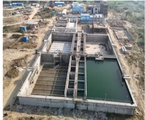
35 MLD STP at Agra
