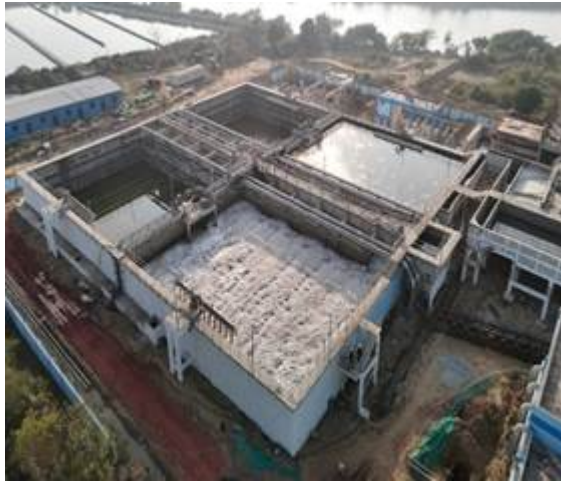
31 MLD STP at Agra
