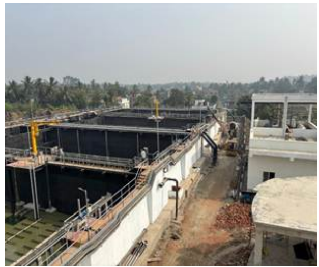
30 MLD STP at North Barrackpore
