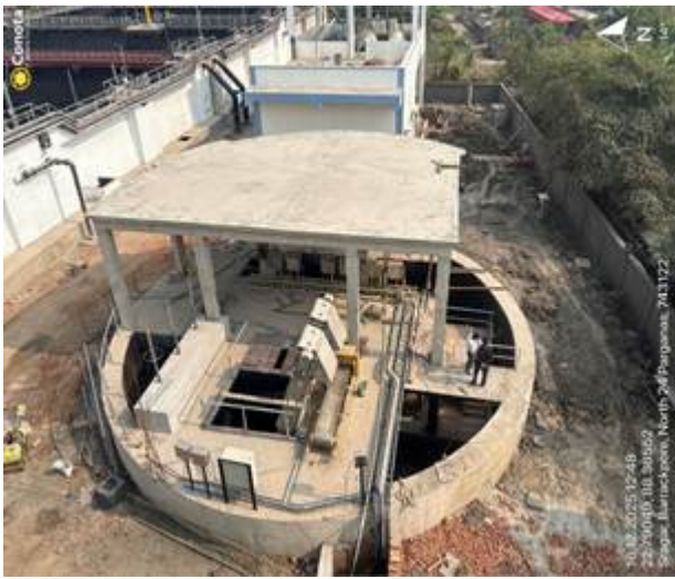
30 MLD STP at North Barrackpore
