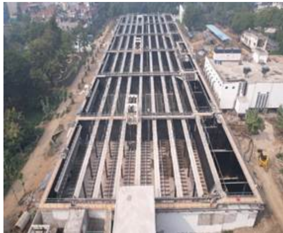
55 MLD STP at Assi BHU, Varanasi
