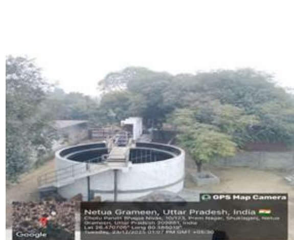
5 MLD STP at Shuklagunj
