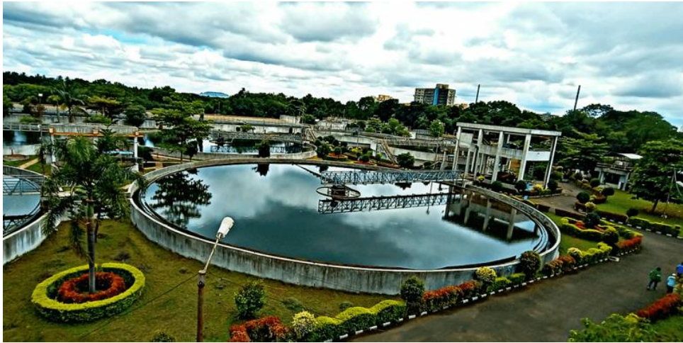
115.00 MLD STP at Naidu, Pune
