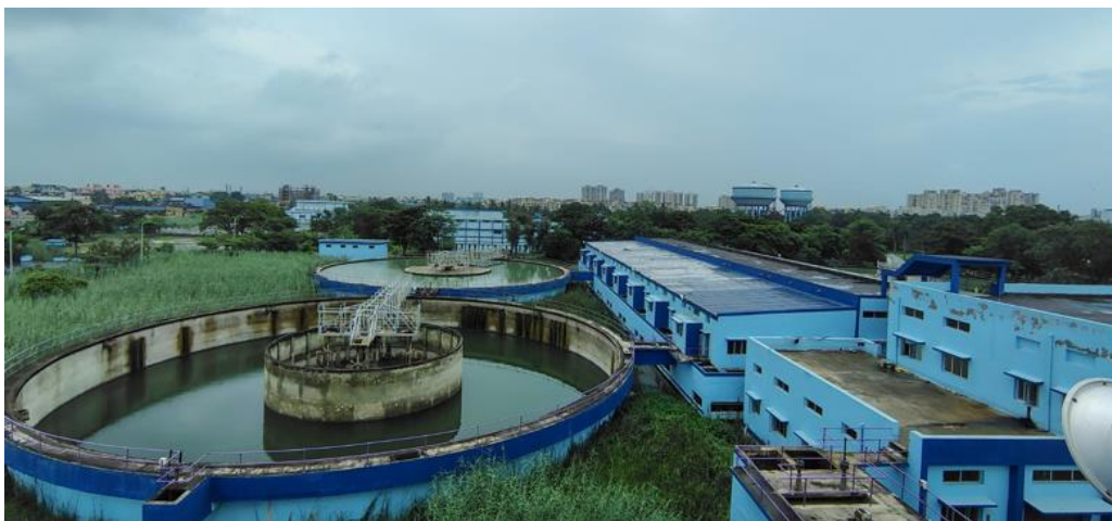
113.50 MLD WTP at Baranagar, Kolkata
