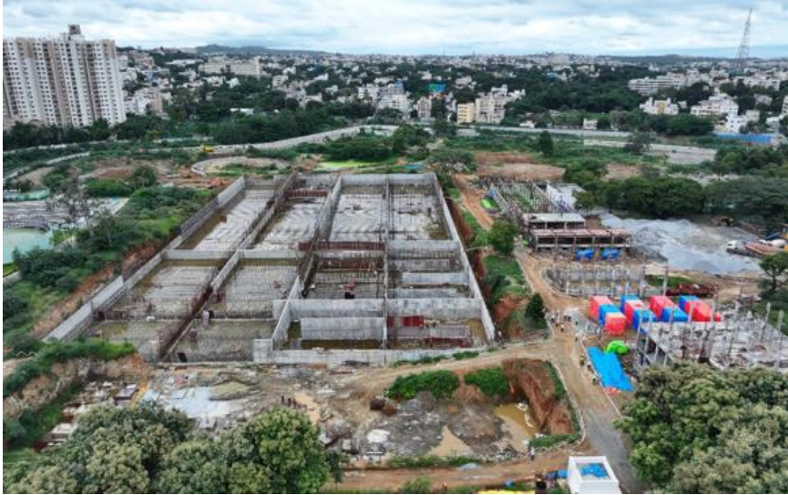
150.00 MLD STP at V Valley, Bengaluru
