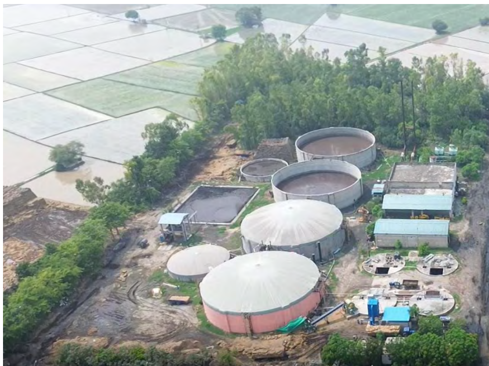
Bio-Gas Generation Plant
