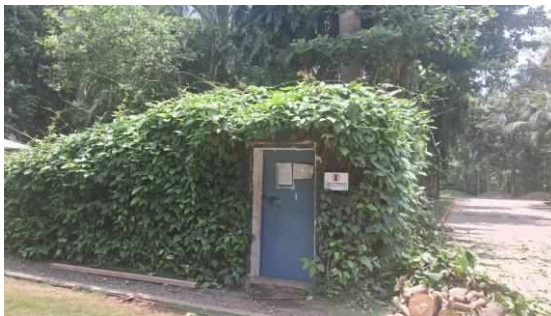
External View of STP in Subject Project
