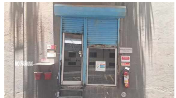
View of HT Room in Subject Project
