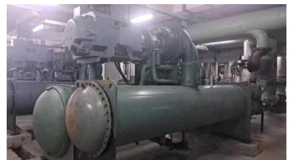
View of Chillers in Subject Project
